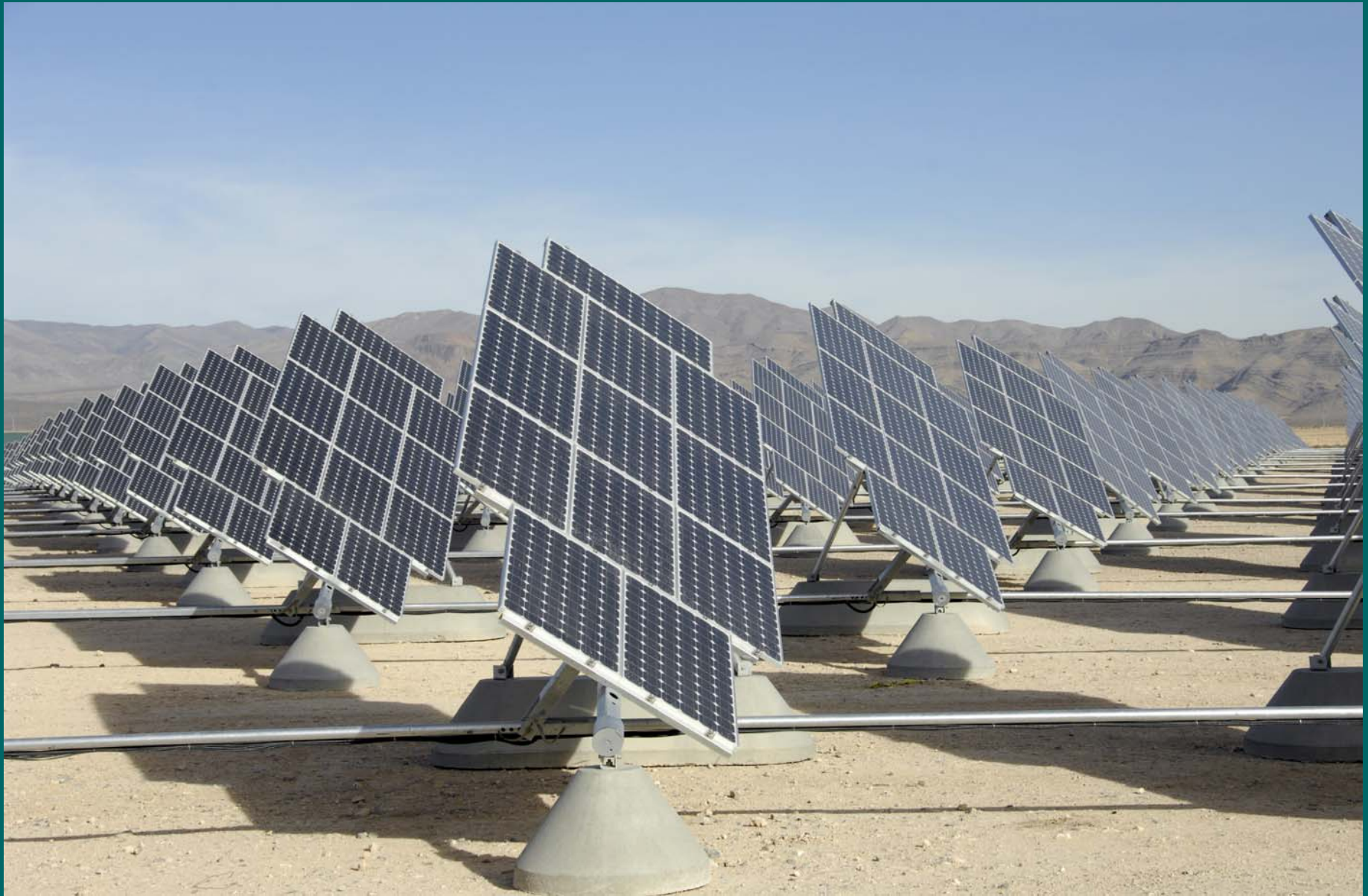
14 MW Nellis Air Force Base – Completed Dec 07
